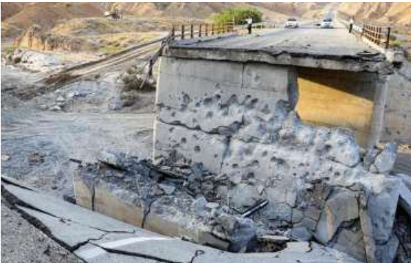
A heavily-damaged bridge which was hit by a U.S. strike along the road connecting Roudan and Bandar Abbas in Iran on Saturday. AFP
