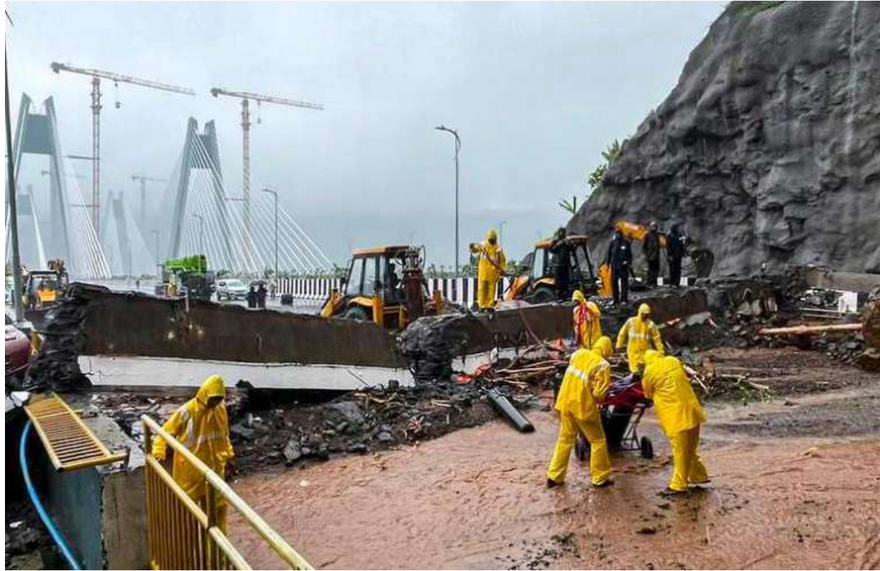
Workers clear debris from the Missing Link section of the Pune-Mumbai Expressway in Maharashtra on Monday, after heavy rain triggered a landslide in the area. The section was opened in May. PTI (REPORT ON PAGE 4)
