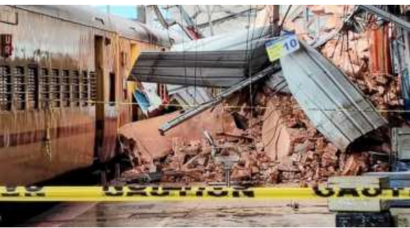
Heavy rain triggered the partial collapse of the 150-year-old heritage clock tower onto Platform No. 2 of the station. K. RAGESH
