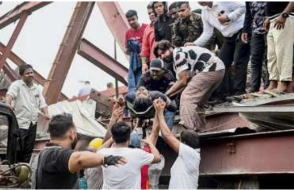
Against the clock: An injured person being taken to safety after a warehouse under construction collapsed in Kolkata. PTI
