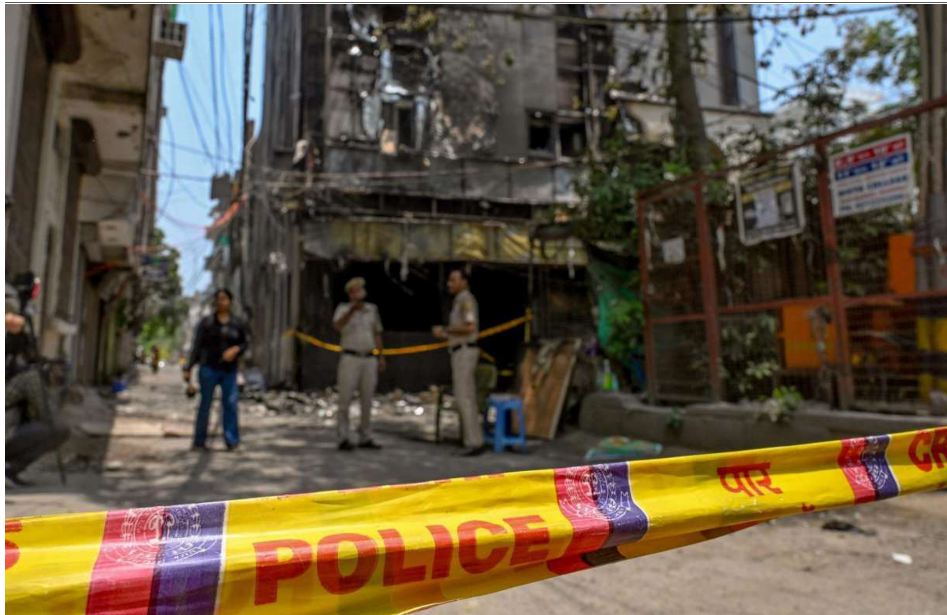
The lane down which Flourish Stay in South Delhi caught fire, where the owner ran a hotel instead of a bed-and-breakfast that the property was licenced for. SUSHIL KUMAR VERMA
