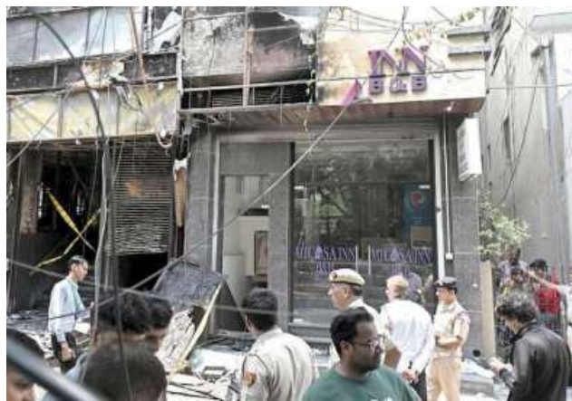
Anxious moments: Police keep vigil outside the entrance of the hotel in Hauz Rani in New Delhi on Wednesday. Some lodgers escaped through windows while local residents helped to carry many of those affected to safety. SHASHI SHEKHAR KASHYAP, AP
