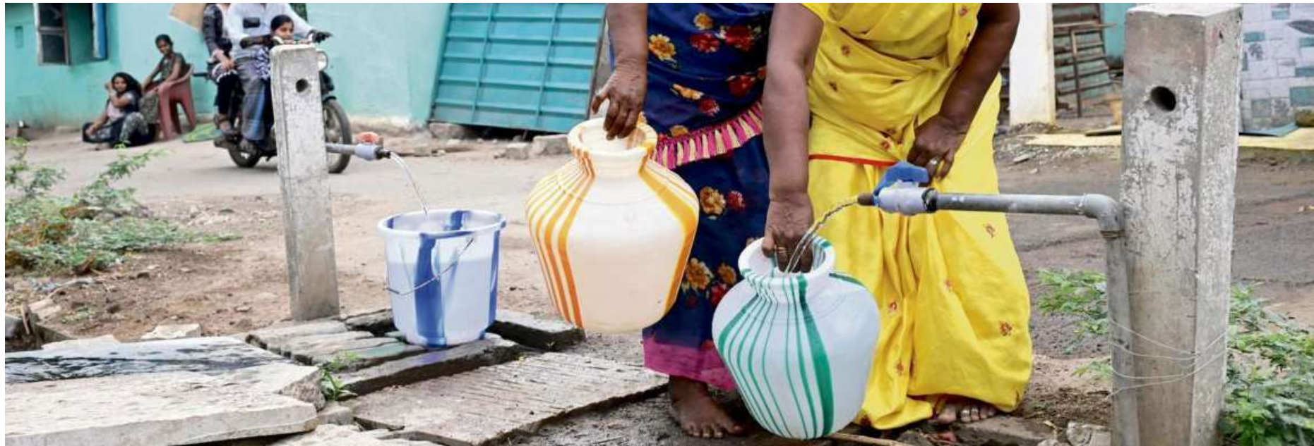
Precious liquid: Women fetching water through the Jal Jeevan Mission water pipes installed at Malaichampuram near Y. Othakadai in Madurai in July. ASHOK. R
